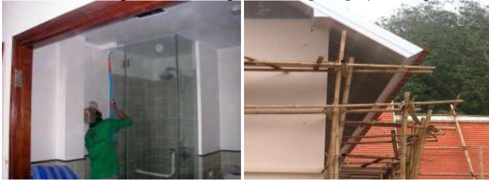
Celing repair Lg1 9B/ the painted barge board on roof and hooks in place for guttering
