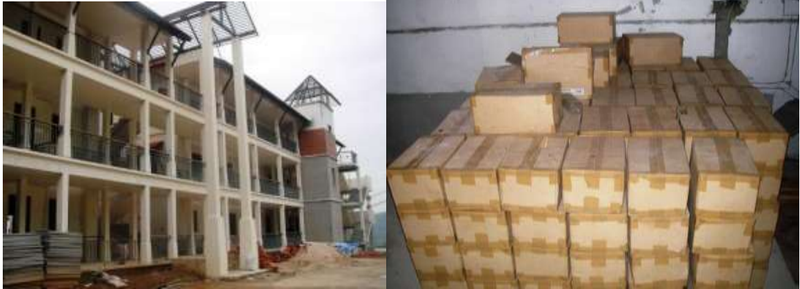
View of back of Lemongrass 2 blocks A and B/Pool tile for the pools with units on this block
