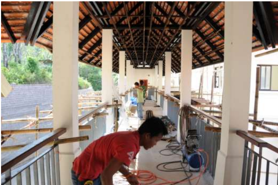
Working on the false ceiling areas of the walkways top level Lemongrass 1
