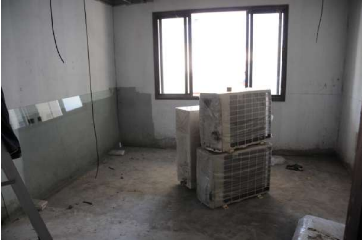
Air Con compressors awaiting installation Lemongrass 2
