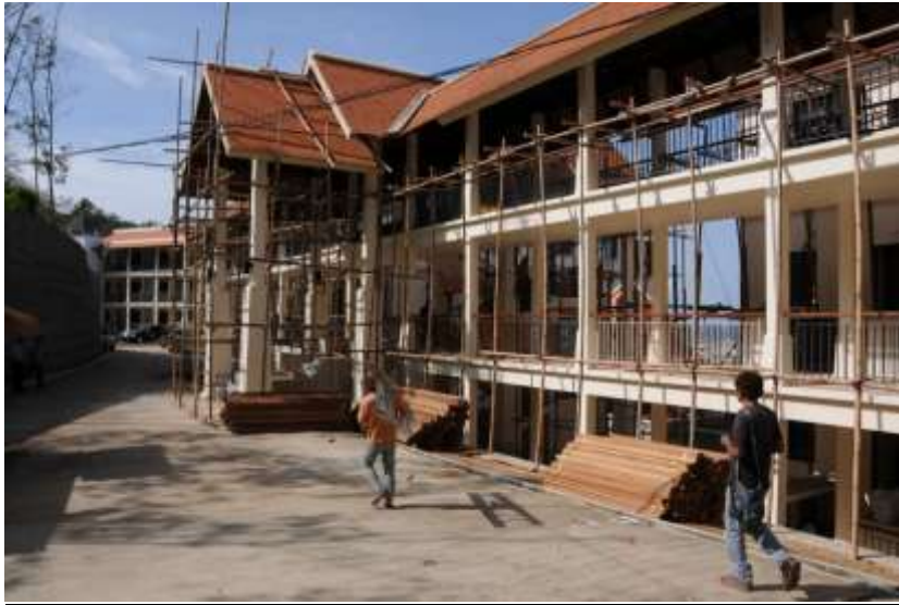
Bamboo scaffold and material for the false ceiling changes to the walkway areas
