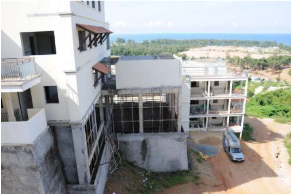
View from Lg 1 to Lemongrass 2 Air con engineer working in extreme front building (green t shirts)
