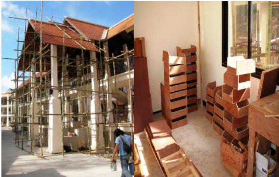
Bamboo scaffolding to commence ceiling work and decoration on walkways Lemongrass1 & stock of drawers under construction in Lemongrass 1
