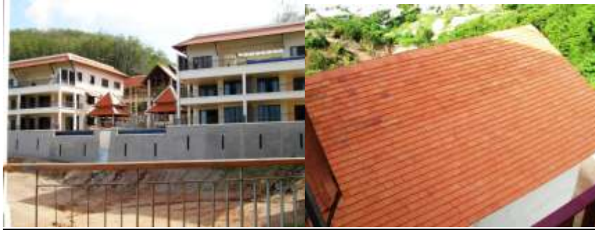
View From LG2 Looking back at LG1 & Roof Tiling work to Lemongrass2 33B
