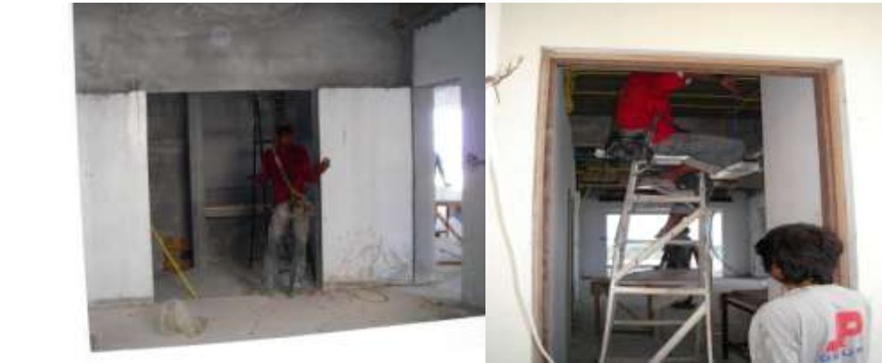
Electric cabling and conduit work in Lemongrass 2 blocks A&B (units 7A &6B)
