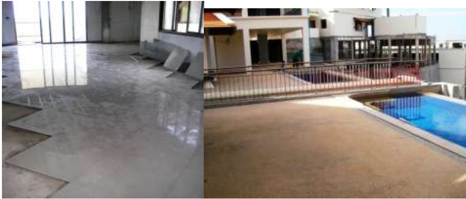
Laying of Tiling in Lemongrass 2 (C&D) and Anti corrosion paint on Lemongrass1 railings
