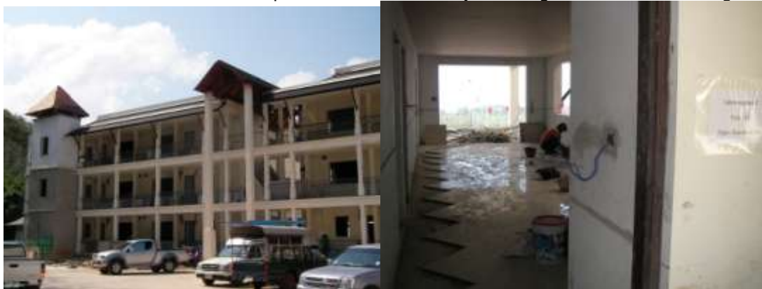
View of rear of Lemongrass 2 A&B Note roof being coloured/tiling of floor in Lg2 11A
