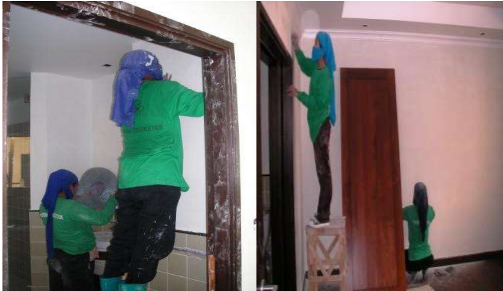
Sanding down fine plaster for smoothing of concrete render Lg1 3A and 8B
