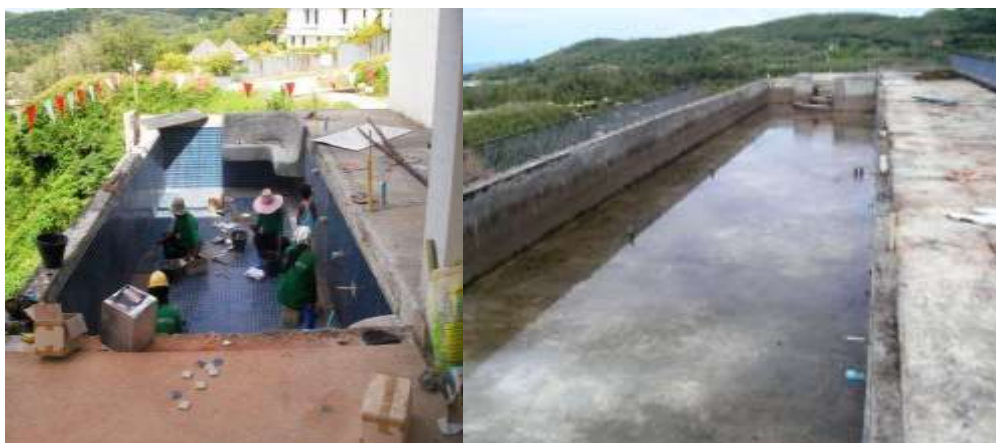
33B pool tile work ongoing and the rooftop pool has been cleaned of the algae.
