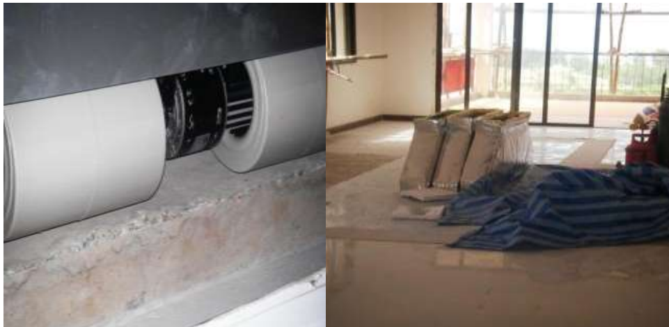
New air handling installed in Lemongrass 1, ductwork awaiting fitting for air con system
