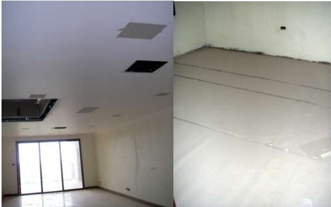
Ceiling rework closing in holes and also protection laid onto flooring where Parquet installed
