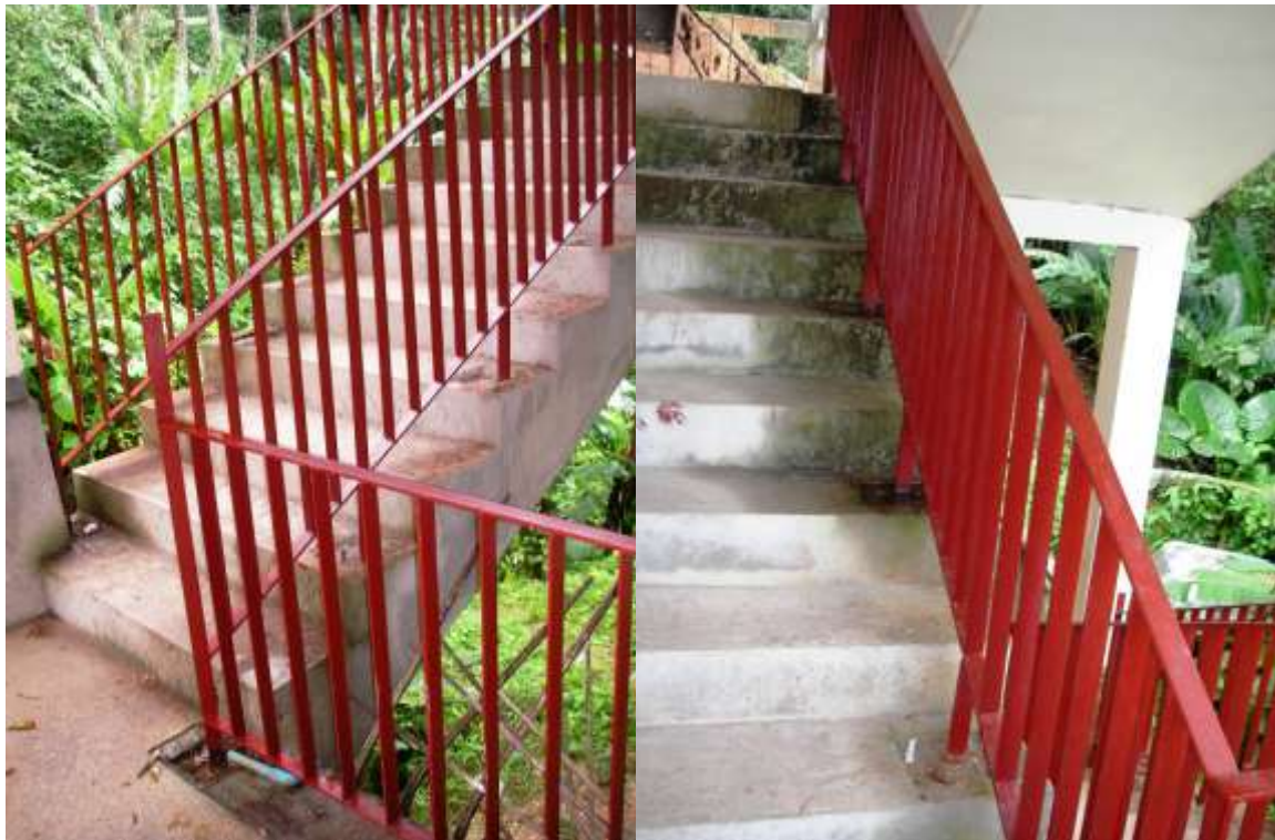
Railings that have been stripped off and repainted with anti oxidant primer ready for final coats.
