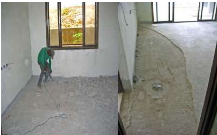
Removing the flooring from previously mislaid cement(previous contractor) so that Parquet flooring can be installed.
