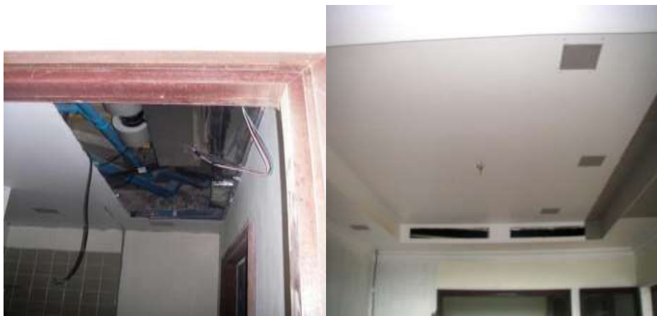
Air handling unit 2 nd bathroom/ reworked ceiling for new circulation from Air con
