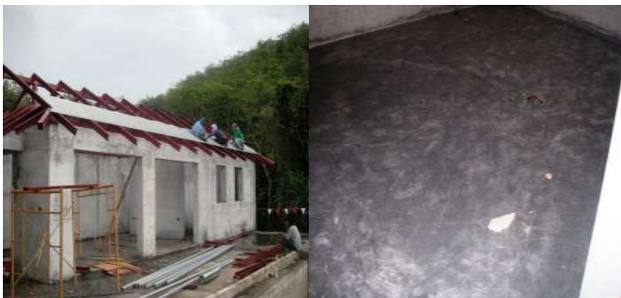
Roofing works on 12c/ relaid cement flooring for the units at correct level for tiling/hardwood floor
