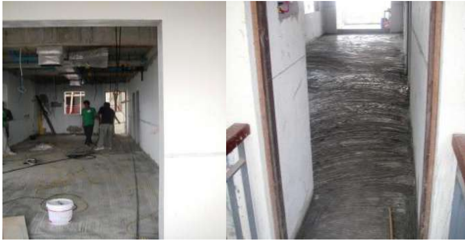
Ongoing rewiring in units and more concrete floor relaid in preparation for tiling.
