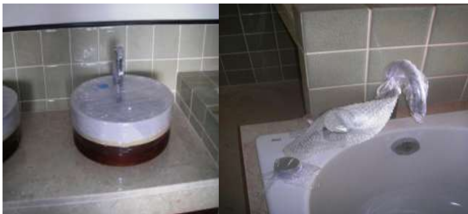
Taps and fittings on basin and bathtub
