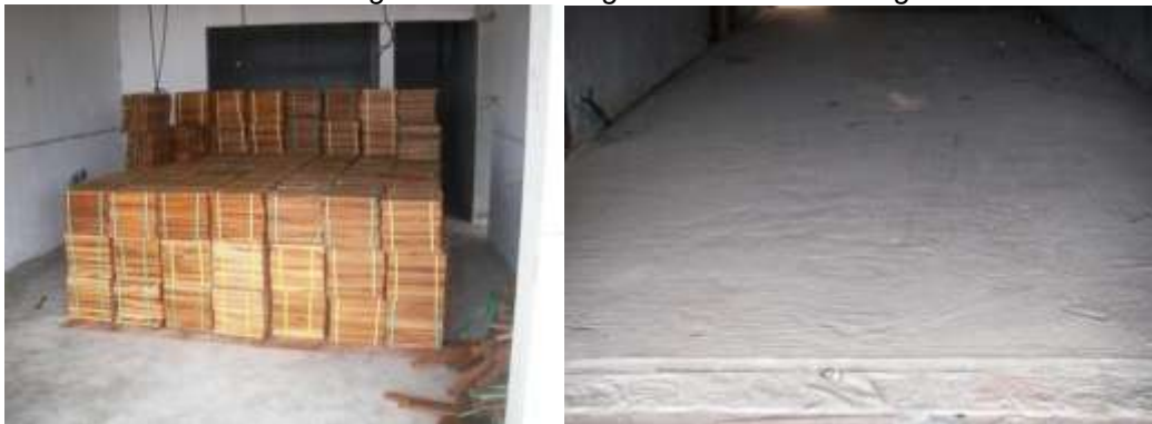
Parquet flooring on site and flooring area prepped ready for ceramic tile (living area)
