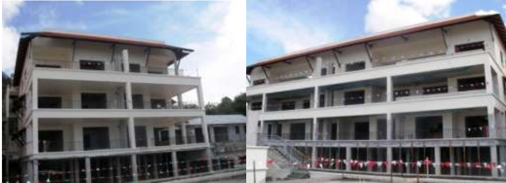
View of blocks A & B Lemongrass 2 from roof garden area of Lemongrass 2 block D
