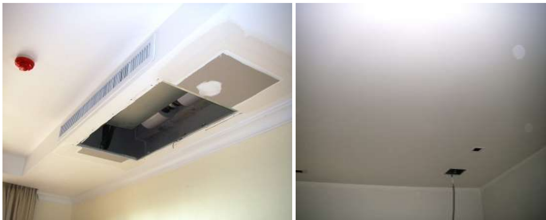
Air handling unit for original showhome replaced/painted bathroom ceilings
