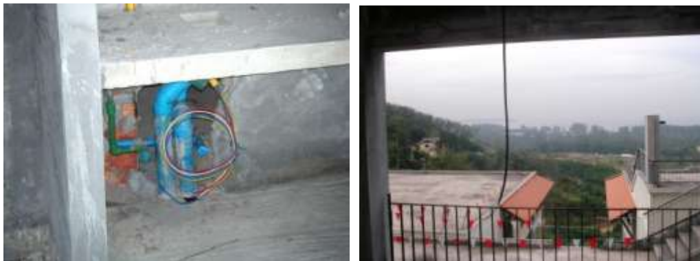
The plumbing rework completed in bathrooms (raise water heater fittings)/view across from 8A
