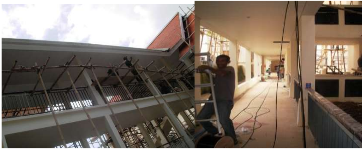
Guttering installed along roof line/ working on cabling of common area walkways
